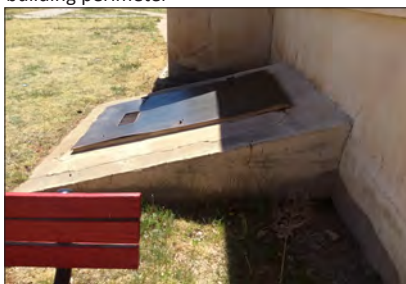
Replace deteriorated entry to basement
