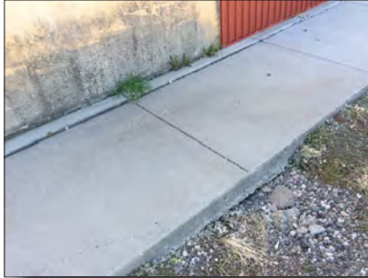
Repair damaged stucco and drainage needs improvement
