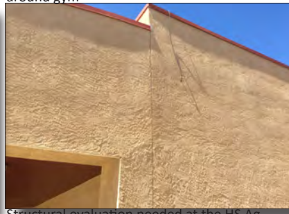
Structural evaluation needed at the HS Ag Classroom
