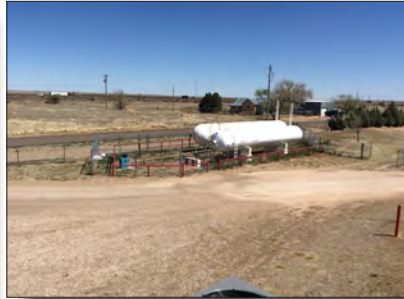
Provide secure fencing around Propane Tank
