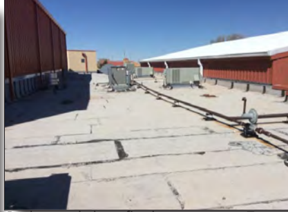
Replace asphalt roofing between gyms. Test rusted gas line connections
