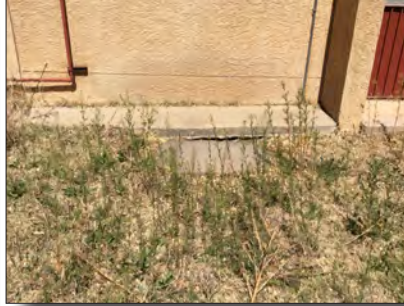
Landscaping improvements needed
