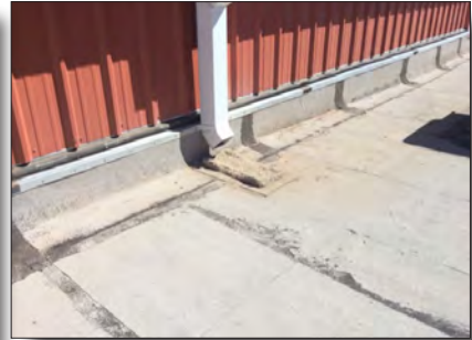
Replace splash-block at downspout.
