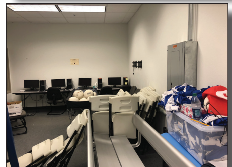
Photos above indicate areas where items are stored in front of electrical panels/ disconnects
