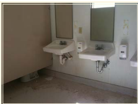
Restrooms are vulnerable to damage and weather
