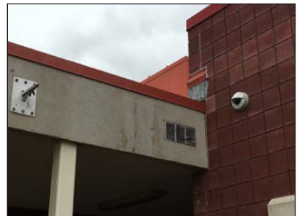
Replace roofing at covered walkway-East side
