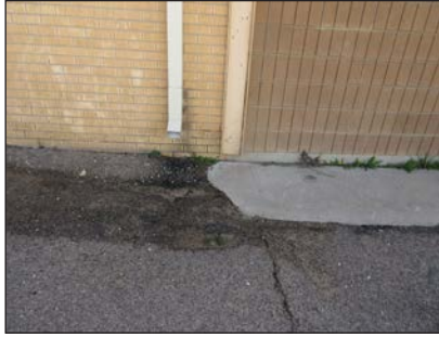
Replace missing downspouts
