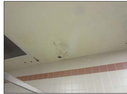
Repair water damaged ceilings in locker room
