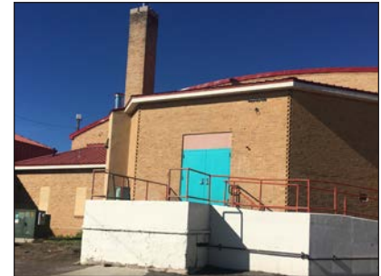
New guard rails needed at delivery dock
