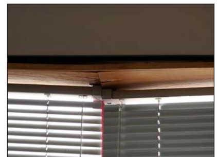
Water damaged window headers
