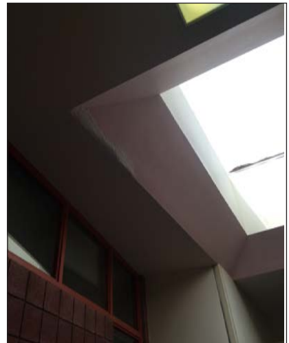
Repair water damage at all skylight wells
