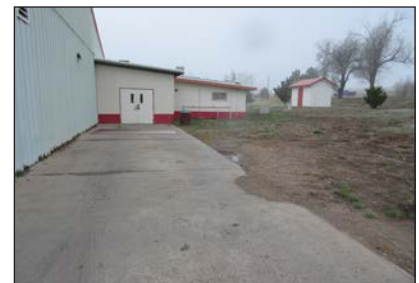
Grading & drainage improvements needed
