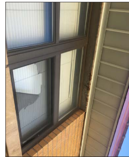
Replace/repair damaged window lintels
