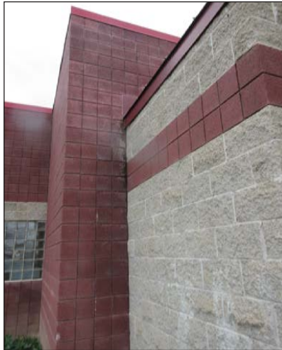
Re-caulk all vertical joints & tuck point masonry
