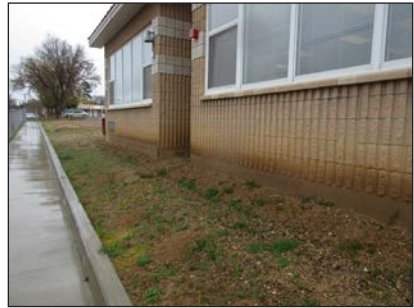
Concrete apron around building needed
