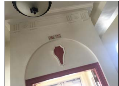
Need Updated Exit Signage
