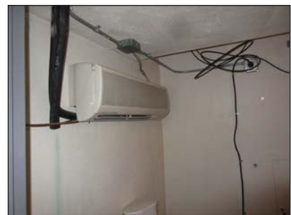
All wiring needs to be cleaned up
