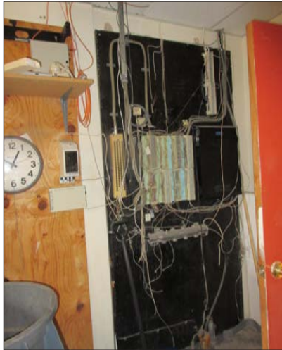
Telephone wiring/cabbling needs to be upgraded
