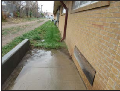
Install concrete apron & splash blocks
