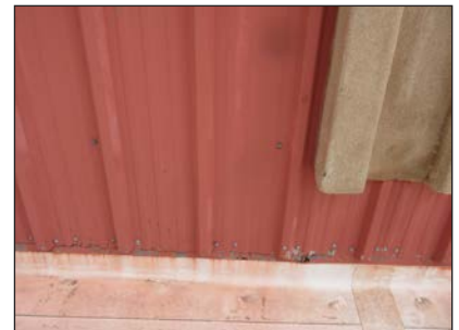
Rooftop metal panels need replacement
