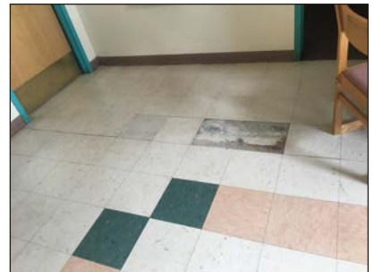
Replace VCT throughout
