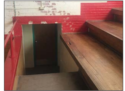
Replace missing handrail-safety hazard
