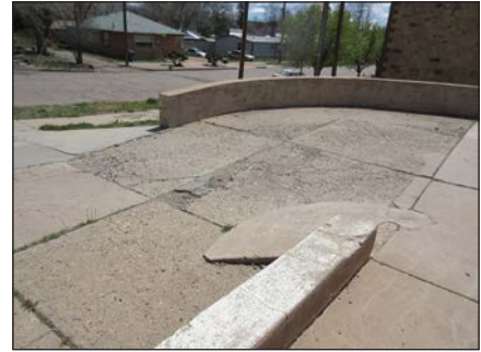
Deteriorated Parking Lot Paving - Rear
