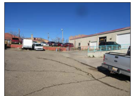
Resurface parking lot
