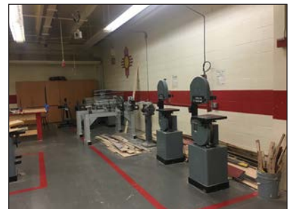
Install Dust Collection System on all Equipment
