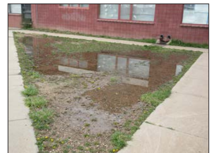
Ponding water - improve drainage
