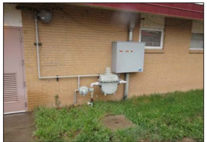
Install concrete apron around building & utility lines
