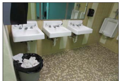
Renovate gym restrooms
