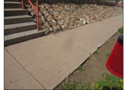
Extend handrails at steps to meet current code requirements
