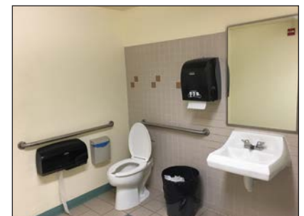
Restrooms renovations needed including ADA compliance
