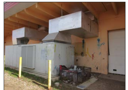
Provide fencing around equipment
