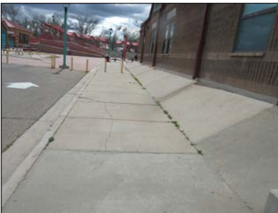
Replace broken/spalled concrete sidewalks
