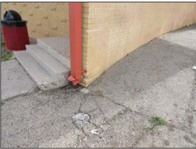
Replace broken/spalled concrete
