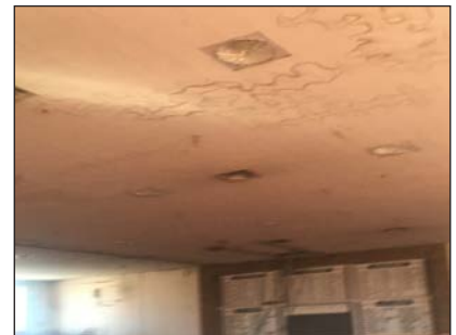
Replace damaged ceiling
