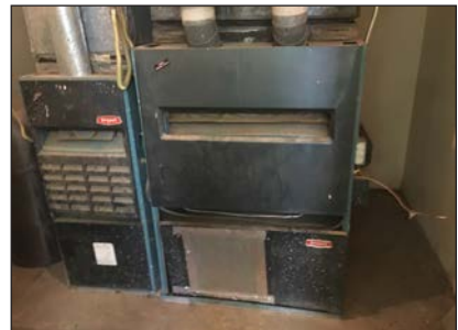
Furnace upgrades needed
