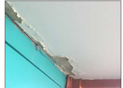
Repair water damage at exterior soffit
