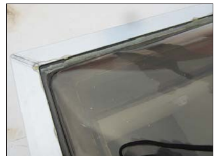
Replace all skylights. Many are broken
