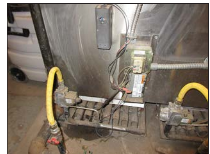
Wiring to be reworked at connections
