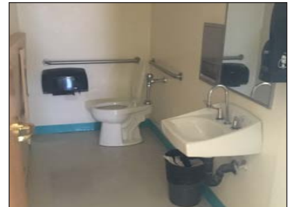
Renovate restrooms for ADA compliance
