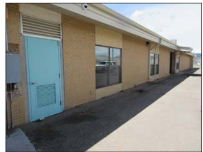
Replace exterior doors & windows
