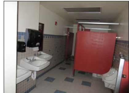
Restrooms need minor refurbishment
