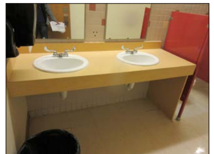
Replace damaged wall tile
