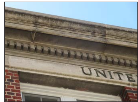
Masonry Restoration/ Cleaning Needed
