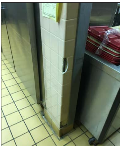
Replace all damaged wall tiles in kitchen
