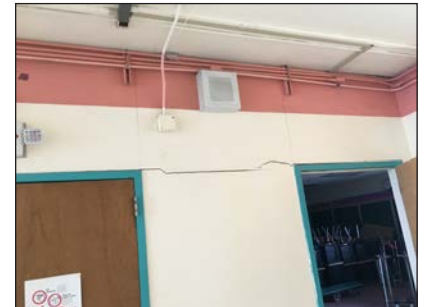
Settlement cracks at NE classroom wing
