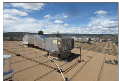
Reroute condensate lines
