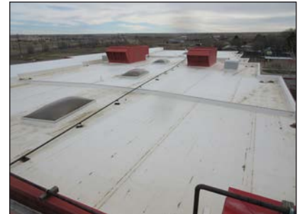
Roof maintenance needed
