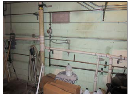
Plumbing upgrades needed
