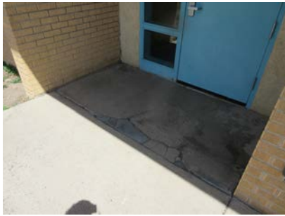
Replace spalled/broken sidewalk
