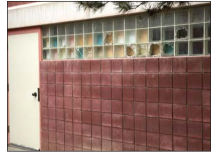
Replace glass block windows
