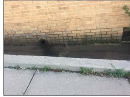
Clear exterior masonry & tuck-point
