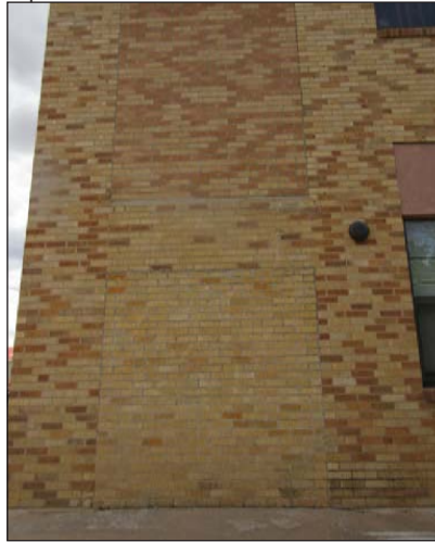
Repair masonry & tuck-point exterior
