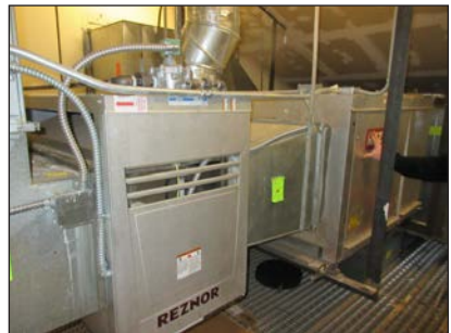
Existing furnace system
