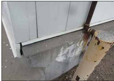
Reseal flashing at all metal wall panels
