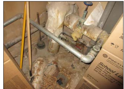
Replace piping insulation
