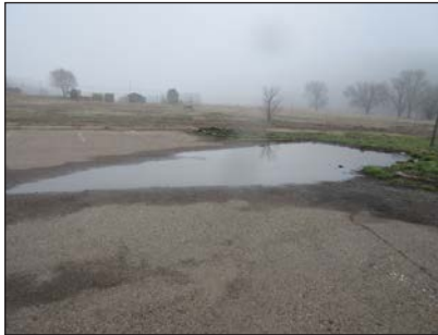
Grading & drainage improvements needed
