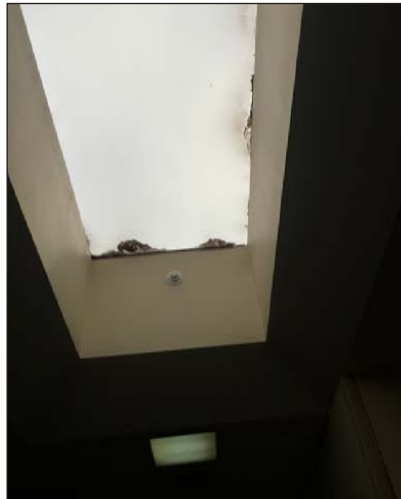
Replace all skylights
