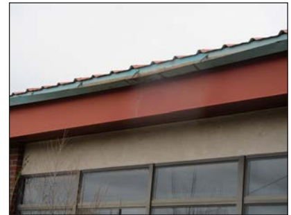
Replace metal roofing/ flashings
