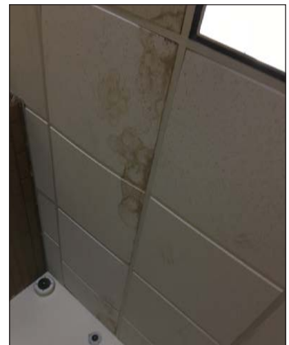
Replace damaged/stained ceiling tiles
