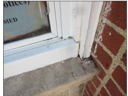
Wood Windows Need Refurbishment/ Caulking
