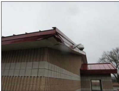
Repair damaged roof corner
