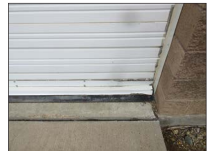
Repair/replace damaged overhead doors
