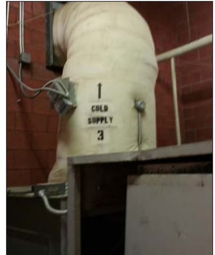
New cooling system needs to be installed
