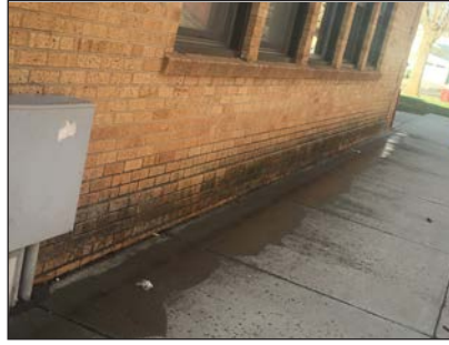
Roof drainage improvements needed on north side of building
