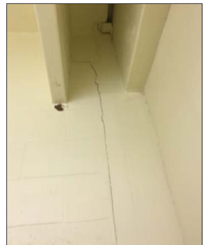
Repair masonry settlement & repaint
