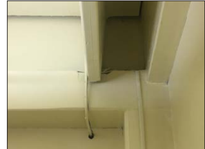
Repair per structural report
