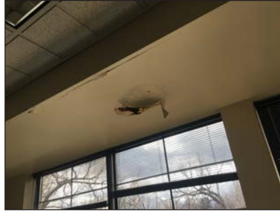
Repair soffits from water leak damage & repaint
