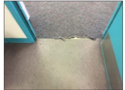
Install transition strip
