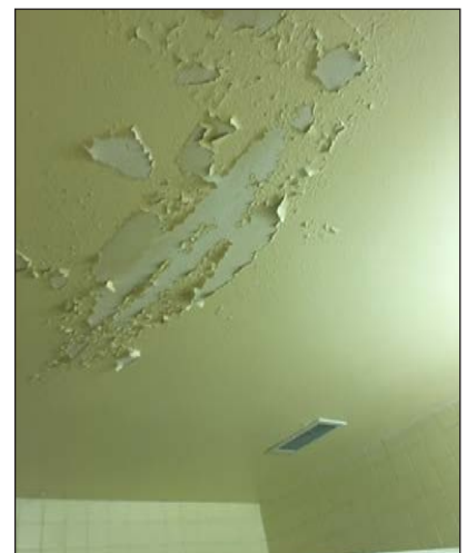
Repair ceilings in all restrooms
