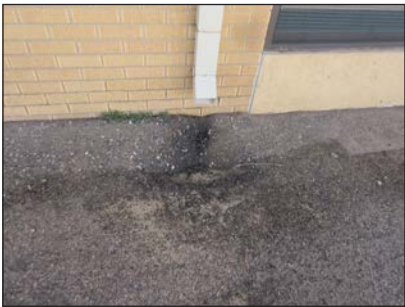
Splash blocks missing
