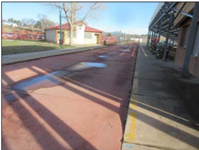
Drainage improvements needed
