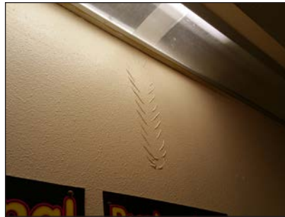
Repair water damaged walls
