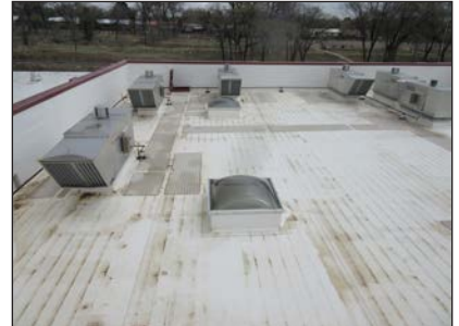
Roof maintenance needed
