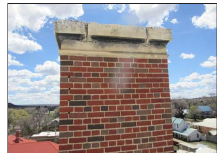
Masonry Restoration/ Cleaning Needed
