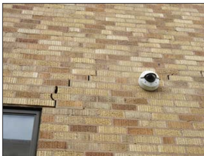
Repair exterior masonry, tuck-point & seal joints
