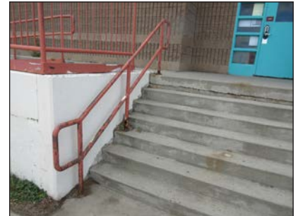
Repaint exterior metal work
