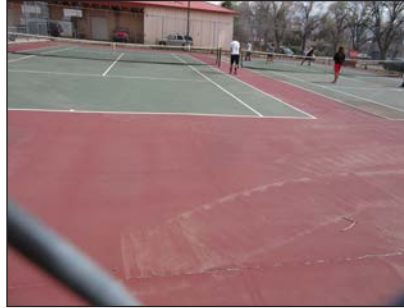
Repair cracks at tennis courts
