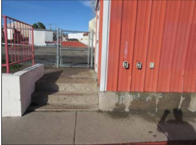
Provide handrails at steps
