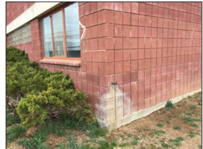
Trim landscaping away from building exterior
