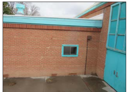
Rework drainage to move water away from building
