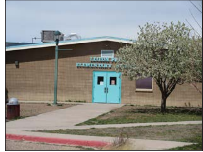
Grading & drainage improvements needed
