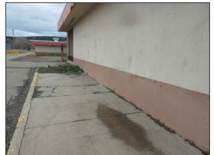
Reseal building perimeter
