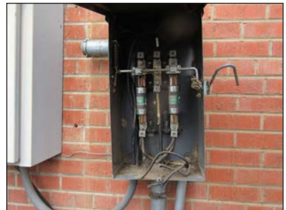
Electrical systems upgrade needed and to be secured
