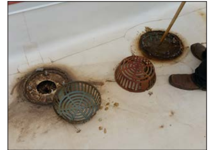
Roof maintenance needed
