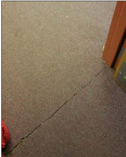
Carpet seams are deteriorating
