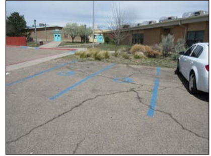
Resurface & re-stripe parking lot to meet ADA requirements
