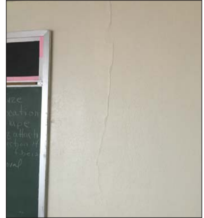
Repair interior wall cracks & repaint
