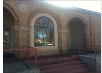
Stairs need handrails installed
