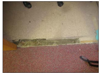
Structural settlement - various locations
