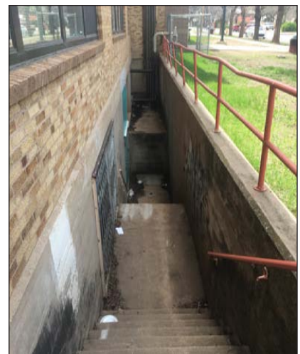
North side: replace basement access stairs
