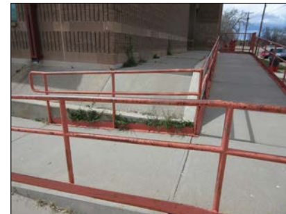
Repaint exterior railings
