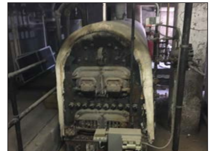
Original Boilers Remain - Non-Operational
