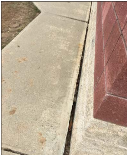
Reseal building perimeter at sidewalks
