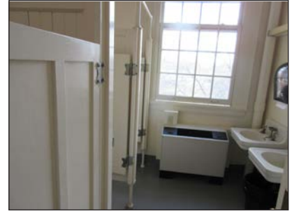
Original 1927 Restrooms - Restoration Needed
