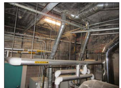
Existing Mechanical System
