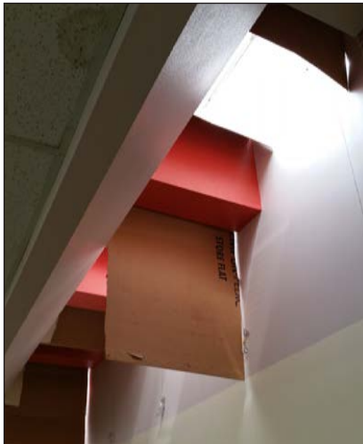
Repair all wall/ceiling water damage at all skylights
