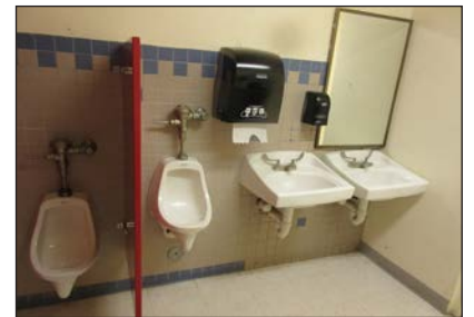
Restroom renovations need to comply with ADA
