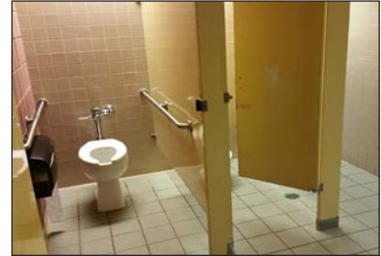
Restroom renovations needed
