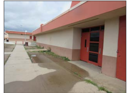
Drainage improvements on west side of gym needed
