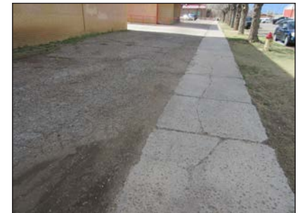
Replace damaged concrete sidewalks & reseal asphalt
