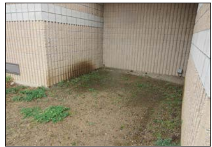
Drainage improvements needed
