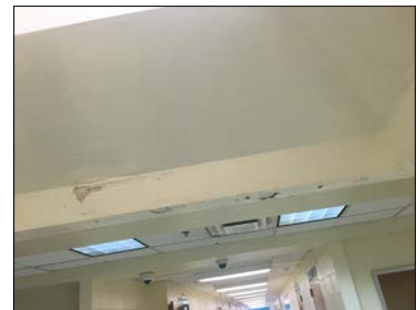
Repair water damaged ceilings & repaint
