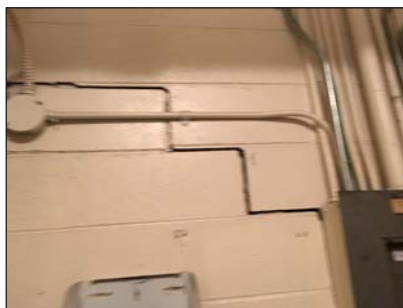
Stabilize & repair structural cracks
