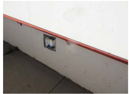
Replace broken ramp lighting
