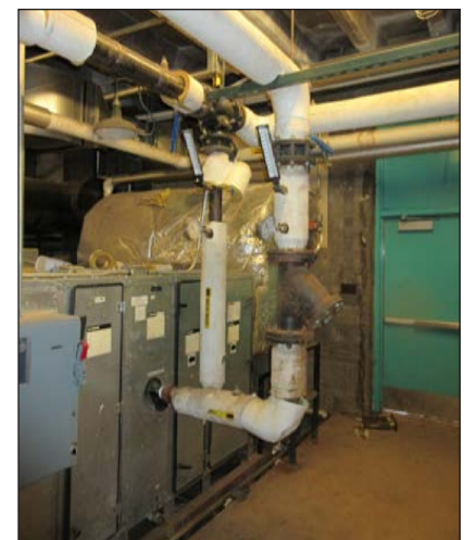
New Boiler System Cooling System Still Needed
