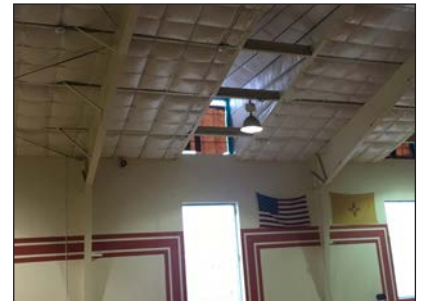
Replace dormer windows with insulated translucent panels to reduce heat
