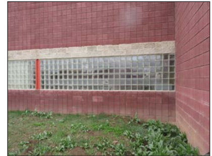
Tuck point masonry & replace glass block
