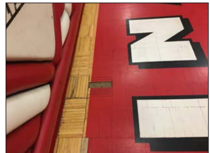
Replace gym flooring
