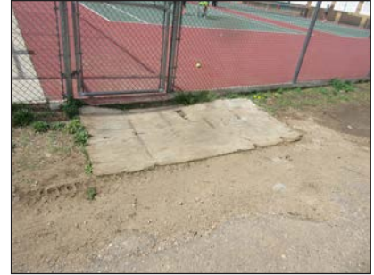
Replace concrete pad & provide sidewalk for ADA access
