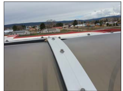
Skylights are in poor condition
