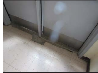
Replace VCT flooring
