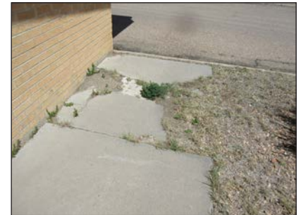
Replace deteriorated sidewalks
