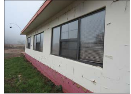
All exterior walls need to be repainted
