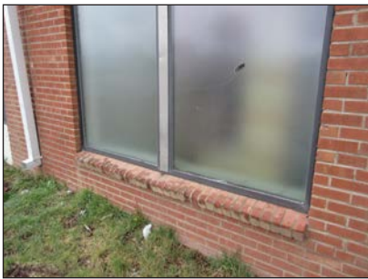
Replace all damaged brick & tuck point masonry
