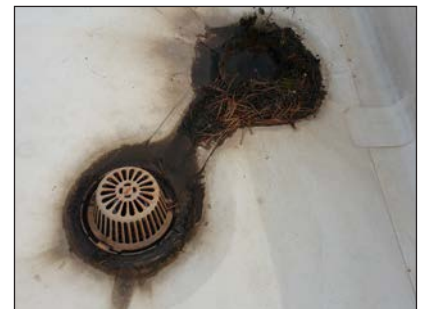
Remove debris from roof drains
