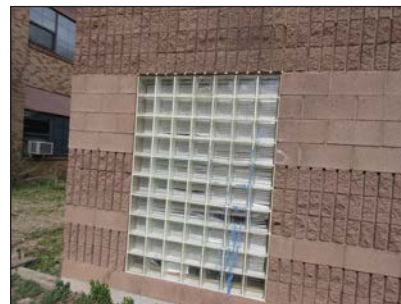
Replace glass block with kalwall system
