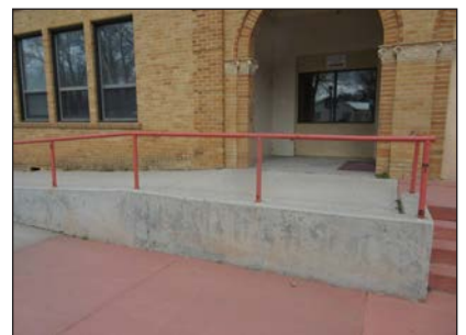
Replace handrails & comply with ADA & current code
