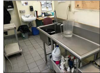
Kitchen renovation needed
