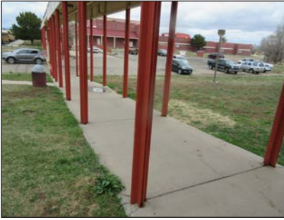
Sidewalk & canopy repairs/replacement needed
