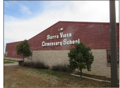
Concrete apron needed around building perimeter
