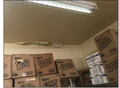
Repair roof leak damage in dry storage room
