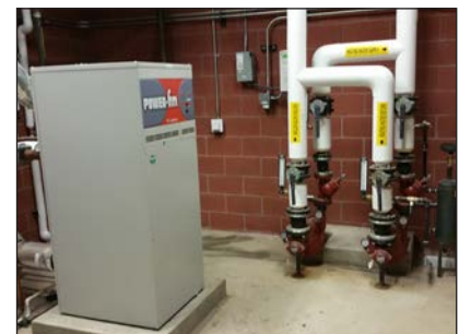
New boiler system
