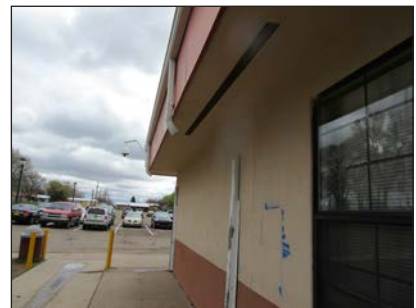
Repair /replace broken downspout
