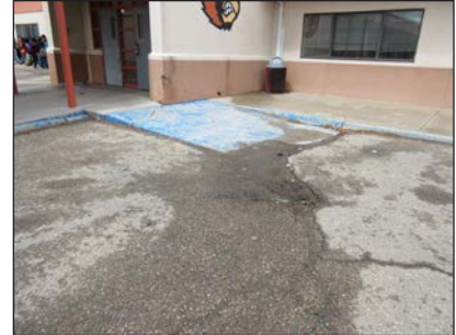
ADA access to the main entrance needs improvement
