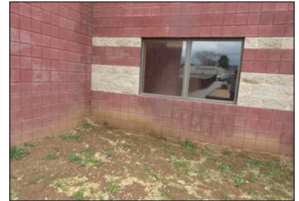
Re-caulk all vertical joints
