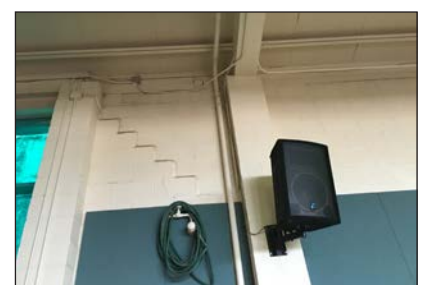
Structural repairs needed in multi-purpose
