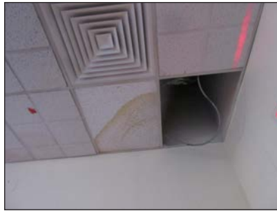
Replace damaged ceiling tiles
