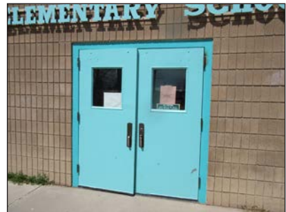
Replace exterior doors & frame
