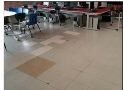
Replace VCT flooring
