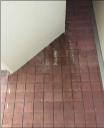
Repair water damage at all walls & soffits
