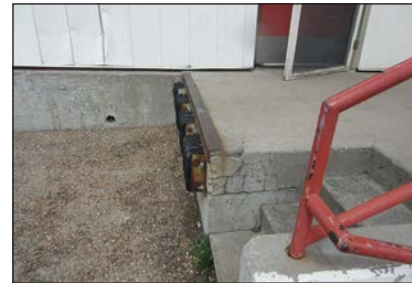
Handrails need to be extended
