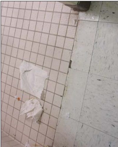
Replace VCT & provide transition strip
