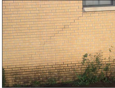
Clear weeds & reseal exterior wall perimeter. Repair masonry & tuck-point
