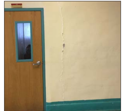
Repair wall damage & repaint
