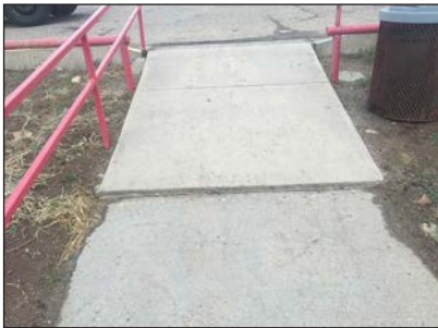
Replace access sidewalk with ADA compliant ramp
