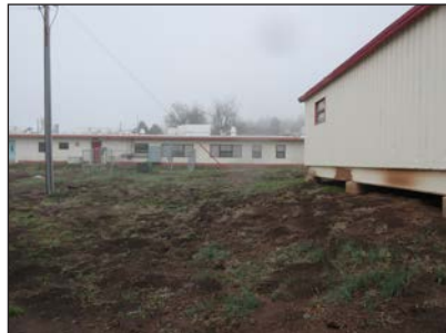
Improve drainage around portables
