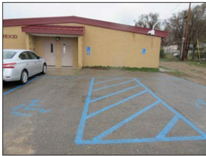
Parking bumpers needed & repave parking lot
