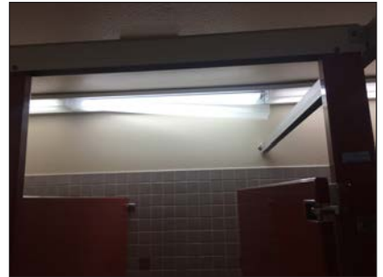
Reattach light lens in restroom
