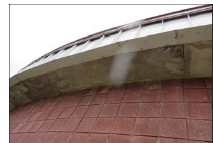
Repair & paint damaged soffits
