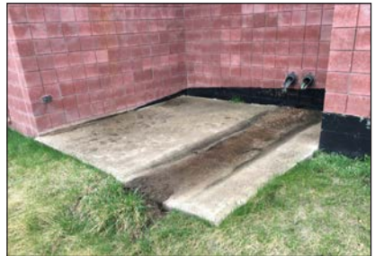
Rework drainage to keep away from building
