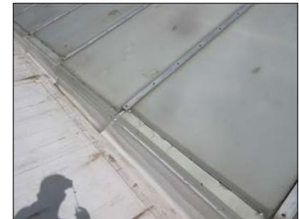
Replace all skylights. Multiple panels broken
