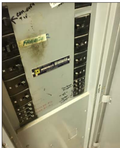
Fix locks/latches to kitchen panels
