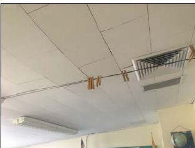
Replace lighting & ceiling system
