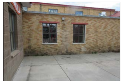
Replace exterior windows & tuck-point
