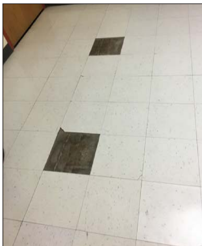
Replace VCT throughout
