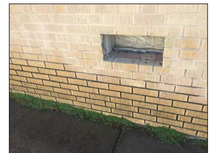
Replace missing exterior vent panel
