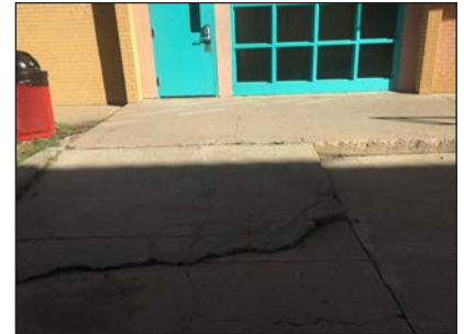
Replace broken/spalled concrete
