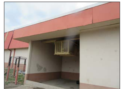
Replace evaporative cooler at kitchen
