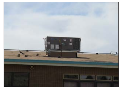
Replace roof jacks
