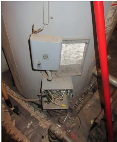
Water heater needs replacement
