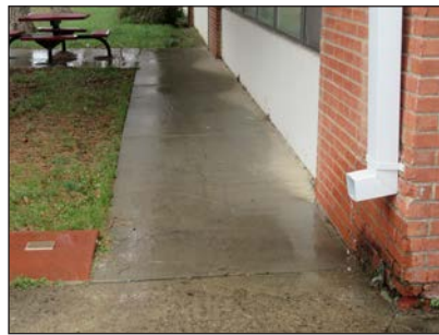
Install missing splash blocks
