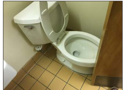
Renovate all restrooms & comply with ADA
