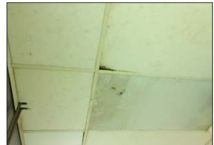
Replace damaged/stained ceiling tiles
