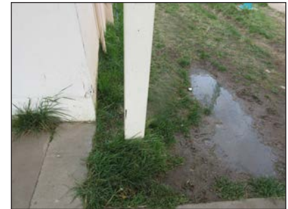
Improve drainage around building perimeter
