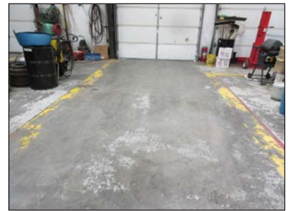
Re-stripe flooring to meet OSHA requirements
