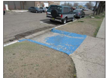
Repaint ADA access curbing/sidewalk
