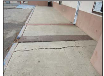
Replace broken/cracked sidewalks
