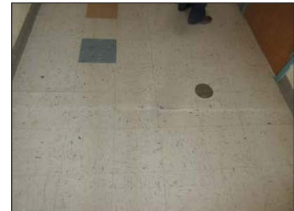
Replace VCT flooring
