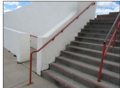
Replace handrails at steps to meet current code requirements
