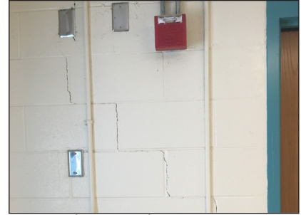
Repair settlement cracks
