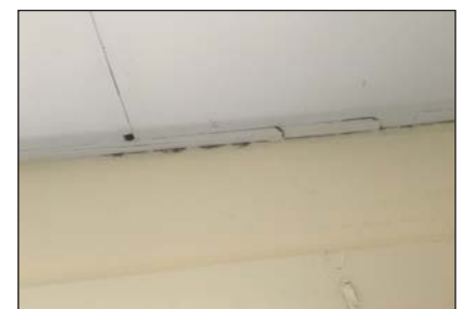
Clean all wall/ceiling joints & repaint
