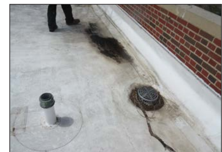
Roof Drains Clogged
