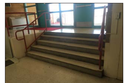
Replace stair nosing's
