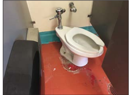
Renovate restrooms & comply with ADA requirements
