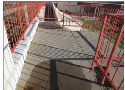
Replace spalled concrete & repaint metal rails
