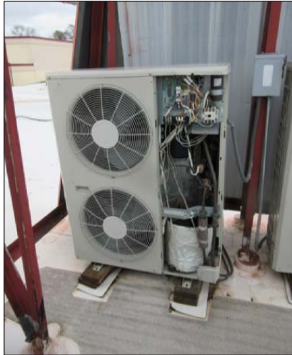
Rooftop equipment needs to be replaced/ repaired
