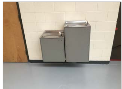
Replace water fountains
