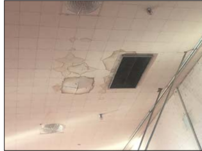
Replace damaged/stained ceiling tiles
