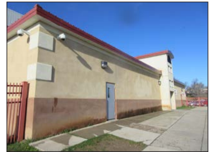
Repaint stucco & re-color coat
