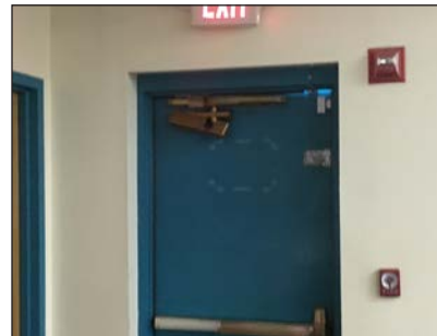
Replace exterior doors & hardware
