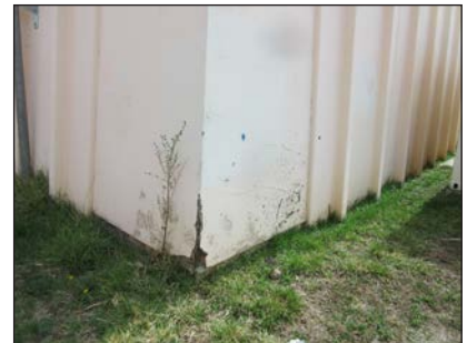
Repair concrete panels & repaint
