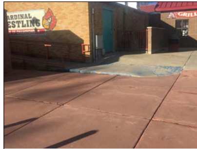
Replace broken/spalled concrete sidewalks
