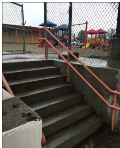
No ADA access to bus drop-off/pick-up
