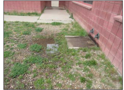
Drainage improvements needed
