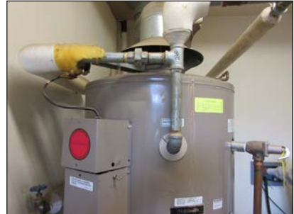
Upgrade & use to new code requirements
