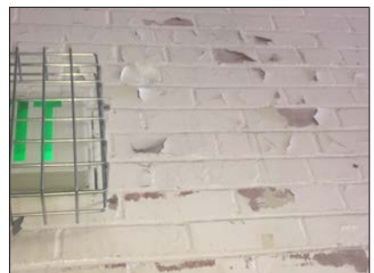
Scrape peeling paint & repaint interior walls
