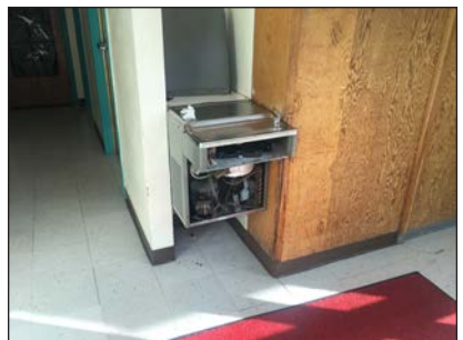
Replace inoperable water fountain
