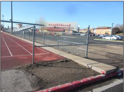
Replace broken/damaged sidewalks
