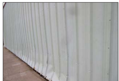
Replace metal wall panels
