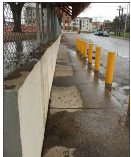
New bus drop configuration needed
