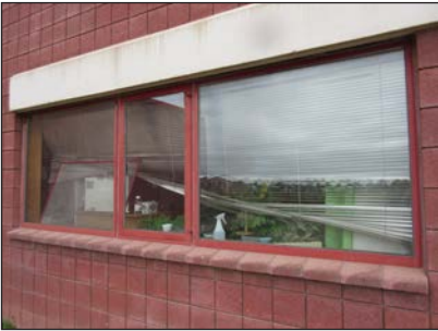
Replace all exterior windows
