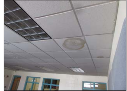
Replace stained ceiling tiles
