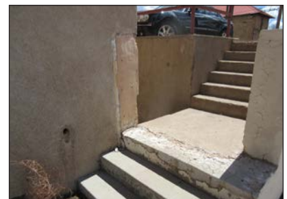
Rear Parking Lot Access Deteriorated Stairs/ No Handrails
