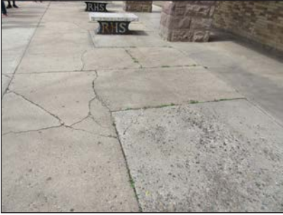
Replace broken spalled concrete
