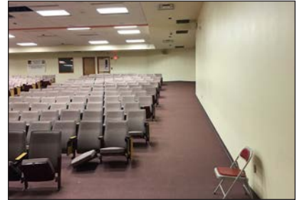
Handrails * landings need to be provided for ADA. Repair/replace seating
