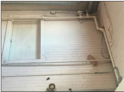
Gym interior needs to be repainted
