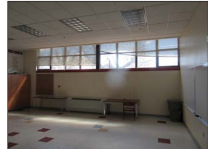
Replace damaged ceilings & upgrade lighting
