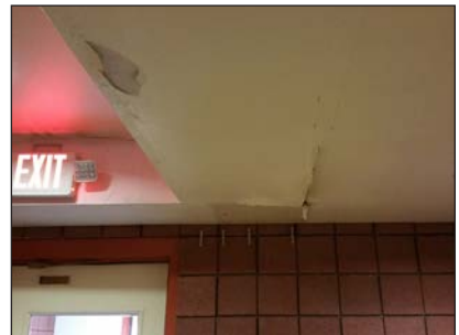
Repair water damaged ceiling
