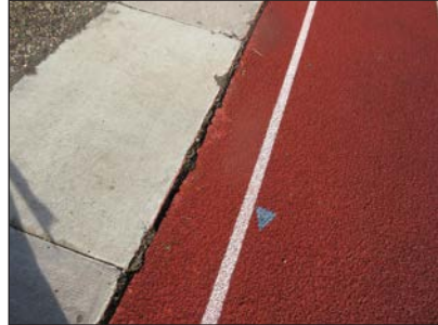
Repair edges around track
