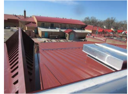
New Metal Roof System
