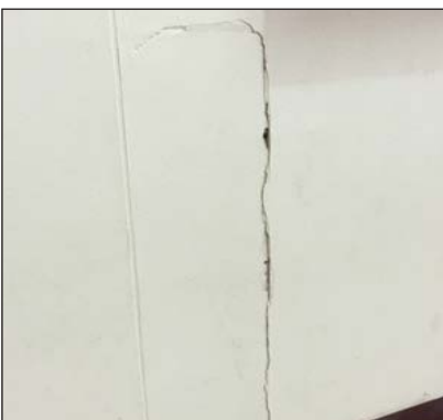
Repair damaged walls in Multi-Purpose room
