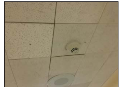
Replace ceiling tiles stained/damaged
