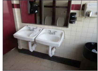
Renovate east restrooms
