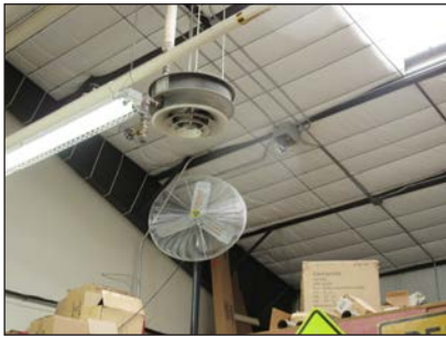
Upgrade HVAC system
