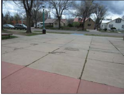
Replace broken/spalled concrete at main entry
