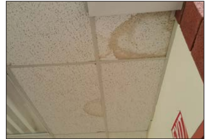
Replace stained/damaged ceiling tiles
