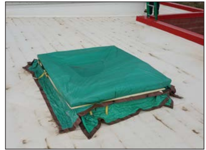
Remove damaged skylight
