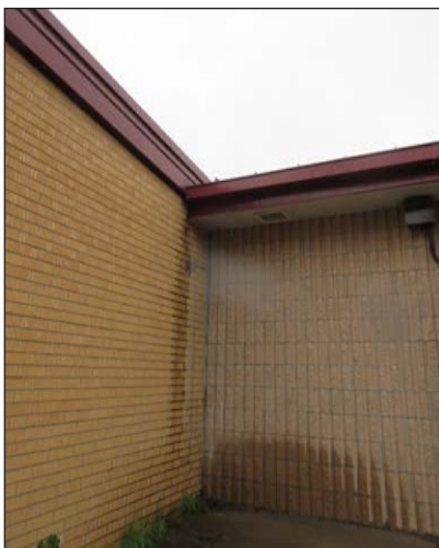
Exterior caulking needed at all joints & tuck point
