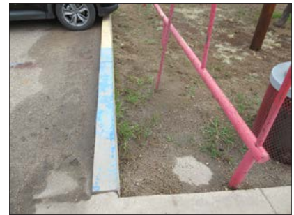
Replace metal railings, repaint curbs & install parking bumpers
