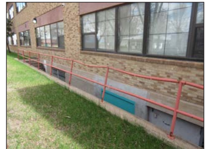
Basement access needs to be redesigned to improve drainage - North side
