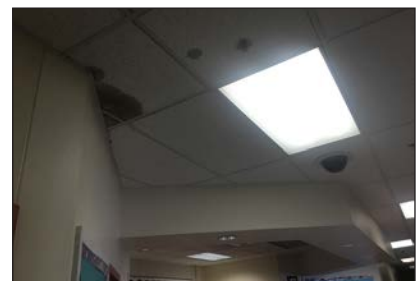
Replace stained/damaged ceiling tiles in admin area
