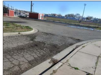
Repair & resurface asphalt
