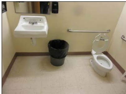
Restrooms need ADA upgrade
