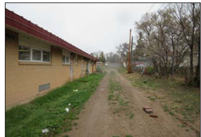
Gutters & downspouts needed
