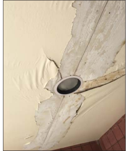
Patch & repair & paint damaged soffit at entrance
