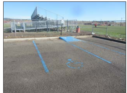
Provide paved surface to access play fields
