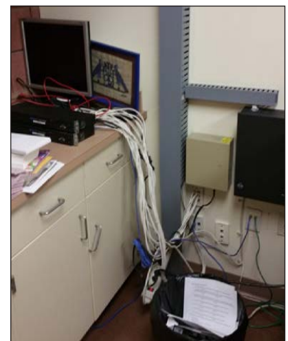
IT wiring & connection clean up required
