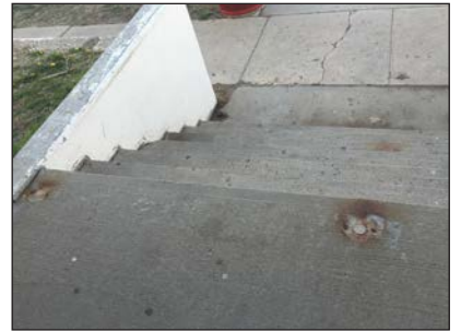
Install handrails at exterior steps to meet code requirements
