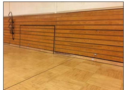
Replace bleachers & comply with ADA
