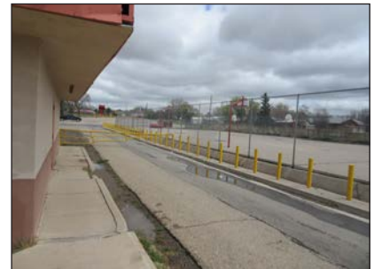
Repave drive lane on south side of gym
