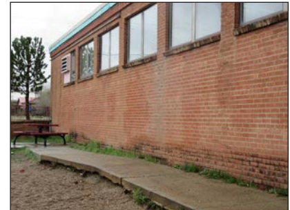
Grading & drainage improvements needed
