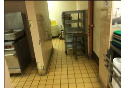
Replace tile & install corner guards
