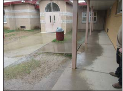
Drainage issues- Regrading needed
