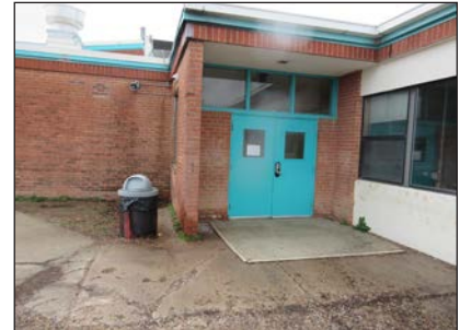
Replace all broken/spalled concrete
