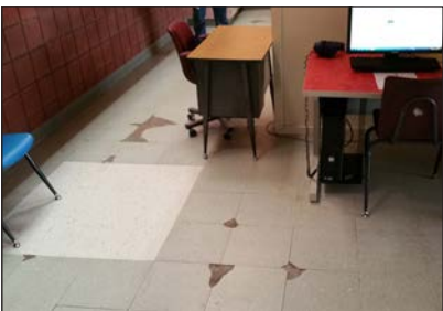
Replace damaged VCT
