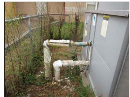
Replace damaged/missing insulation
