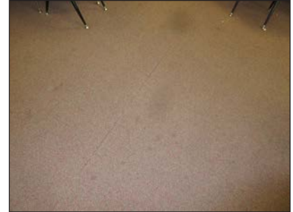
Replace carpet tripping hazard
