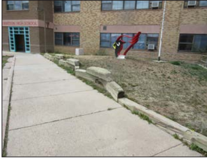
Replace damaged/spalled concrete sidewalks
