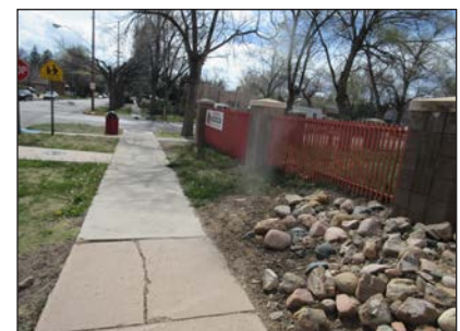
Replace broken/settling sidewalk
