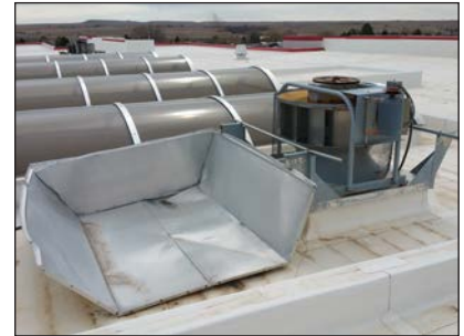
Reattach covers to equipment
