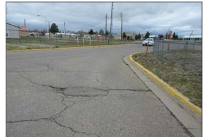
Resurface parking lot
