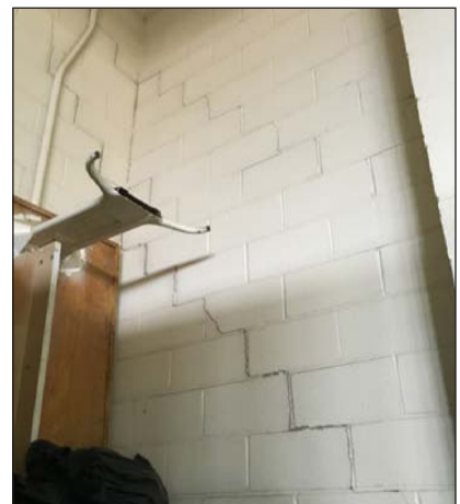
Extensive wall cracks in gym
