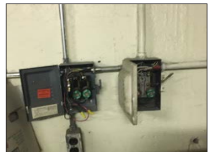
Original Panels Remain With Glass Fuses
