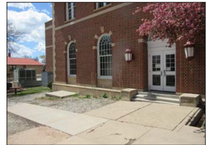
Side Entrance to Building - Broken Sidewalks
