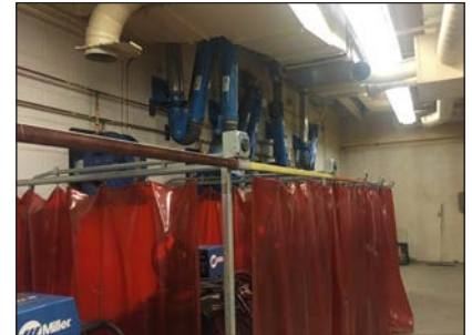
Replace all welding equipment hoods - Non Operable System
