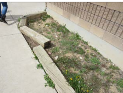
Reset/replace R.R. ties
