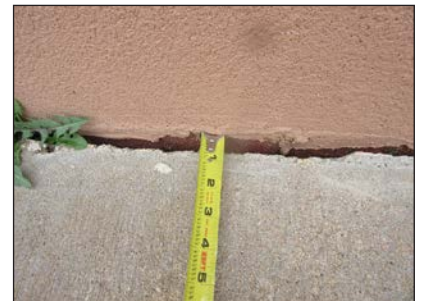
Settlement occurring-see structural report. Reseal wall base around perimeter
