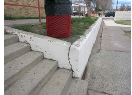
Repair retaining wall & provide handrails at steps
