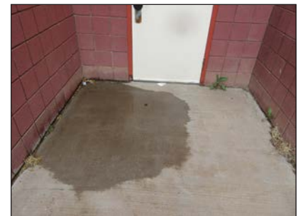
Replace rusted doors & frames & reseal at concrete base
