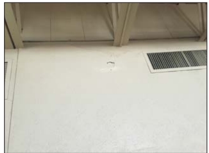
Repair interior walls & repaint
