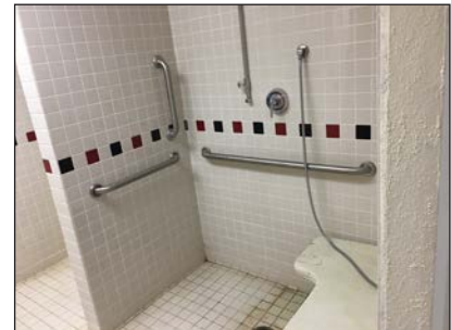
Repair ADA shower & provide curtain
