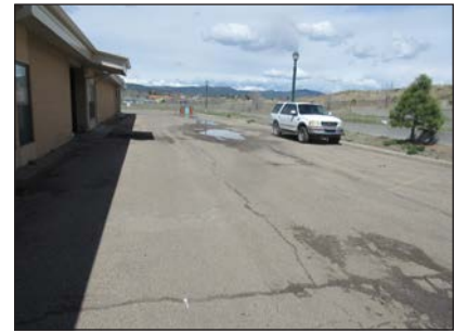
Resurface paving on northeast side of building
