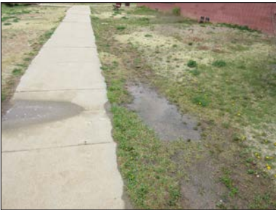
Replace damaged/spalled concrete sidewalks
