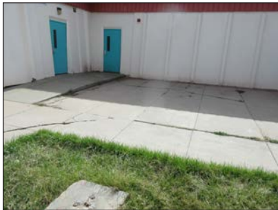
Replace broken/settling sidewalk
