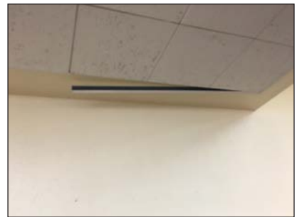
Replace HVAC system
