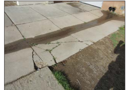
Replace broken sidewalks
