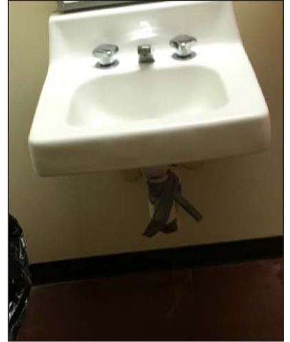
Renovate all restrooms & comply with ADA requirements
