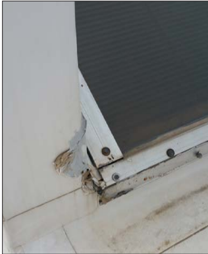
Damaged roof flashing at all skylights
