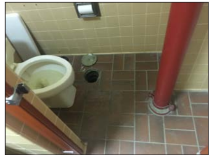
Non-accessible toilet area (3rd level)
