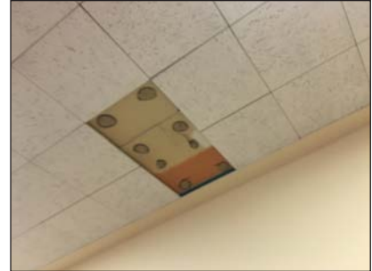
Replace missing ceiling tiles
