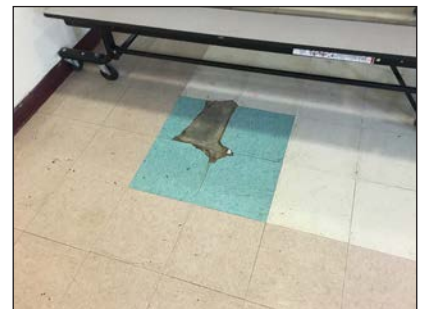
Replace VCT in multi-purpose room
