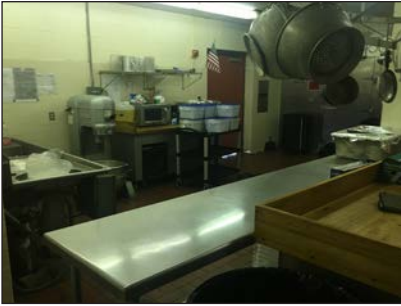
Complete kitchen renovation needed
