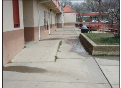
Site drainage issues between main building & gym
