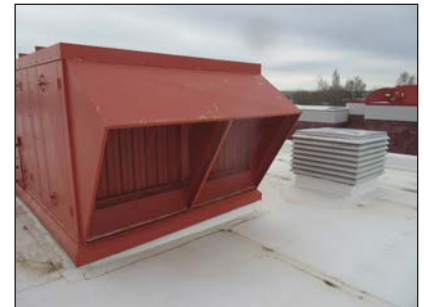
Air handlers need to be upgraded
