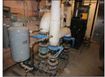
Replace boiler system
