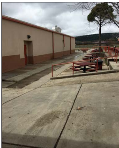
Drainage gutter/culvert needs to be replaced for positive flow
