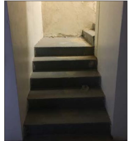
Handrails need to be installed at stairs
