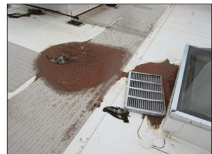
Remove debris & equipment on roof
