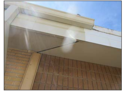
Repair/replace metal flashing
