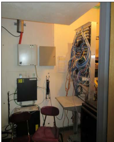
IT server & equipment needs to be reorganized
