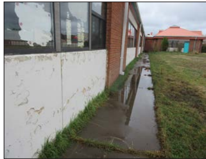
Remove loose paint at concrete panels, reseal & repaint
