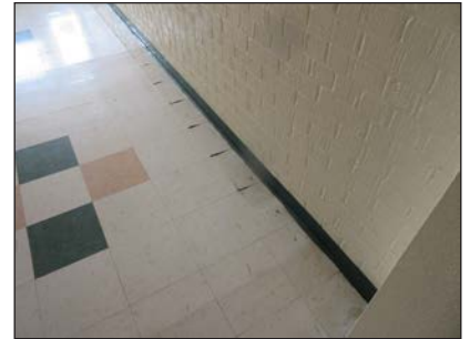
Replace VCT flooring
