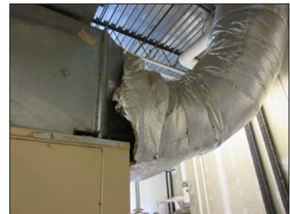
Ductwork insulation needs to be repaired/ replaced
