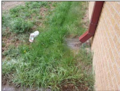
Reset splash block for proper drainage
