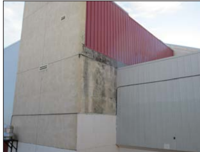
Reseal all vertical joints including metal panels
