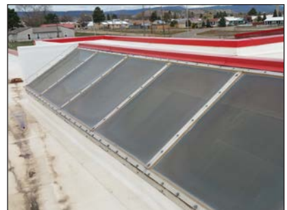
Skylight seals failing
