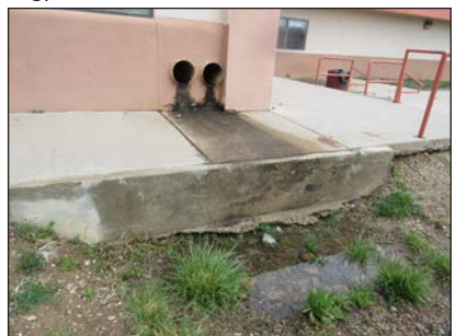
Regrade site & replace sidewalk. Provide under sidewalk roof draining
