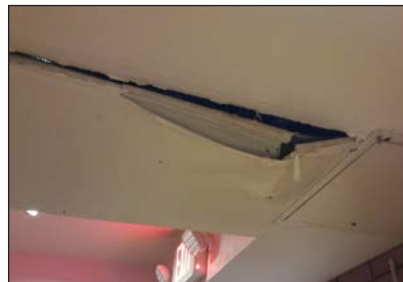
Patch repair & paint ceiling
