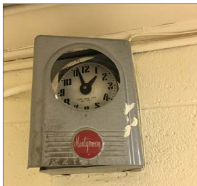
Replace original school clock system
