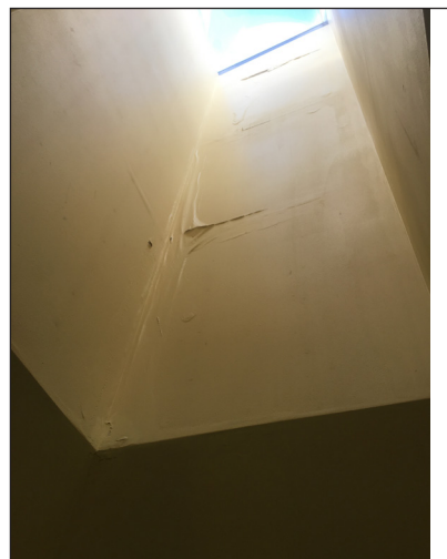
Repair water damage at skylight wells
