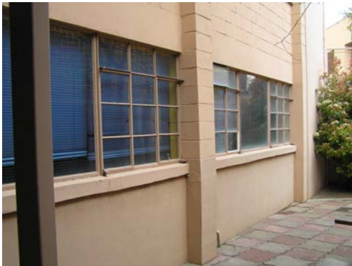
Although windows provide great day lighting to the classrooms, the current materials also contribute to some energy inefficiencies.
