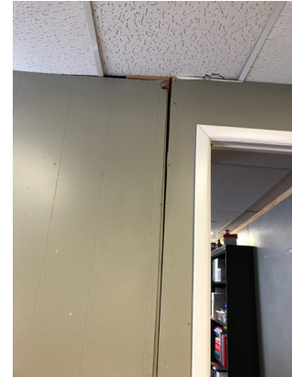
Seam inside portable (gap)
