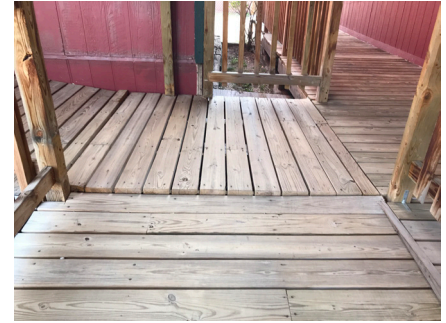
Walkway with tripping hazard
