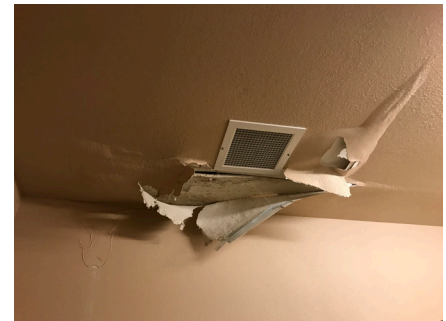
Ceiling at restroom damaged from roof leak
